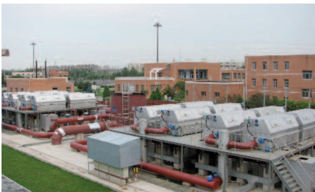
River and sea outfall application in China: 16 ROTAMAT® Rotary Drum Screen RoMesh® units with 0.2 mm square mesh for wastewater treatment
