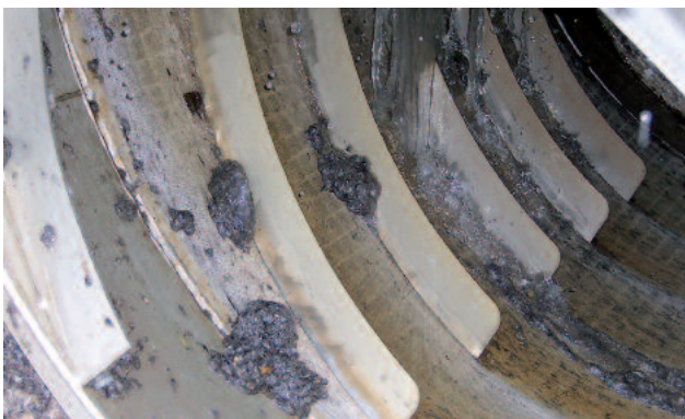
River and sea outfall application: wastewater screening with a ROTAMAT® Rotary Drum Screen RoMesh®
