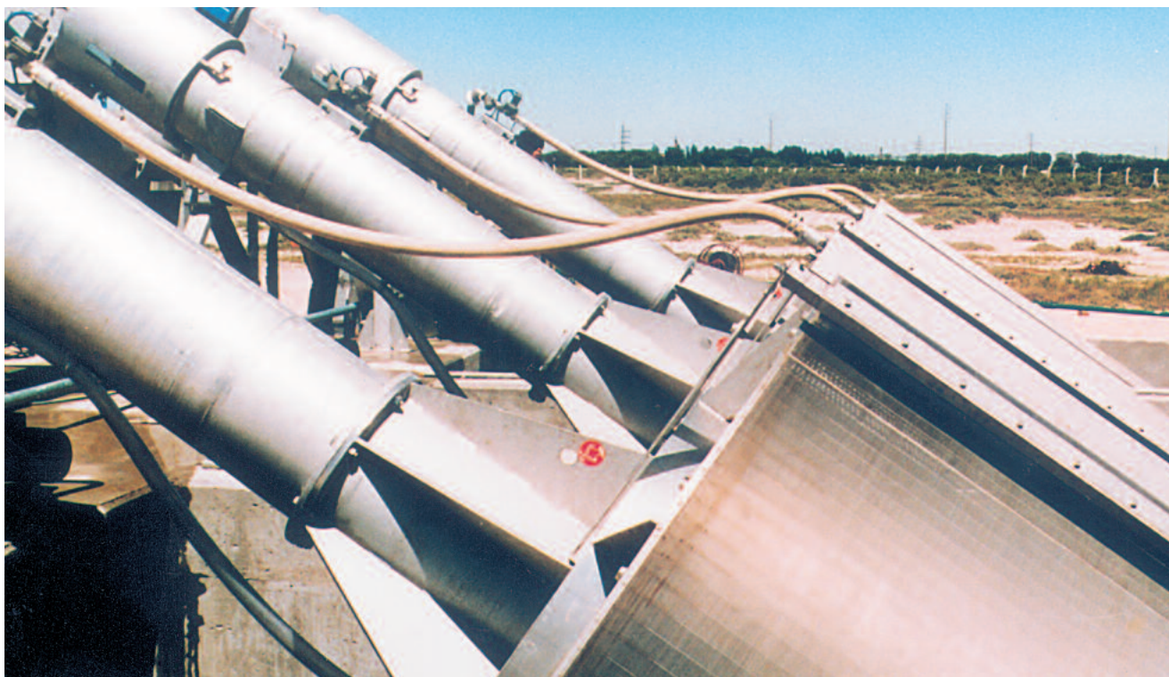
Bahia Blanca, Argentina: Three ROTAMAT® Wedge Section Screens installed in the channel ensure odour-free dewatering and removal of the screenings and significantly improve this river and sea outfall application
