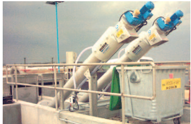
Outdoor installation of a ROTAMAT® Rotary Drum Fine Screen Ro 2 with insulation
