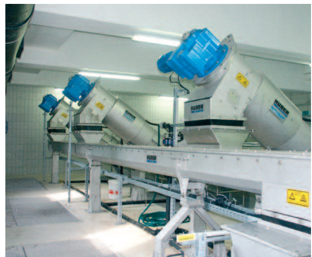
Wastewater fine screening with three ROTAMAT® Membrane Screen RoMem units
