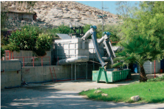
Wastewater screening with a 2 mm ROTAMAT® Rotary Drum Fine Screen Ro 2
