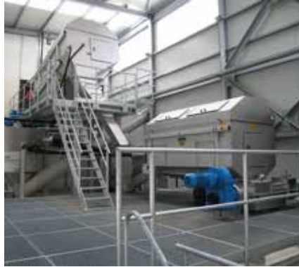
Complete treatment system for sewer grit and road refuse.
