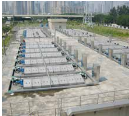
24 installed HUBER Disc Filter RoDisc® units.
