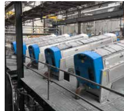
Sludge dewatering with HUBER Screw Press Q-PRESS® 800.2.
