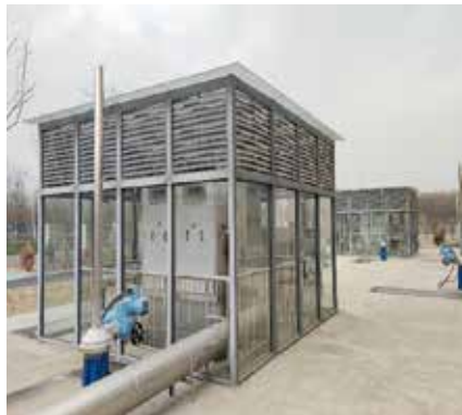
HUBER Band Screen CenterMax® HF as second stage of drinking water treatment.
