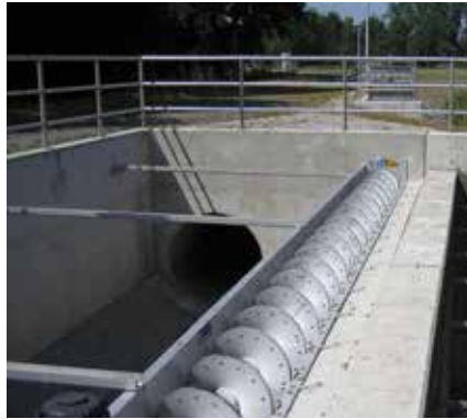
HUBER Storm Screen ROTAMAT® RoK1 installed on dry side of overflow weir.
