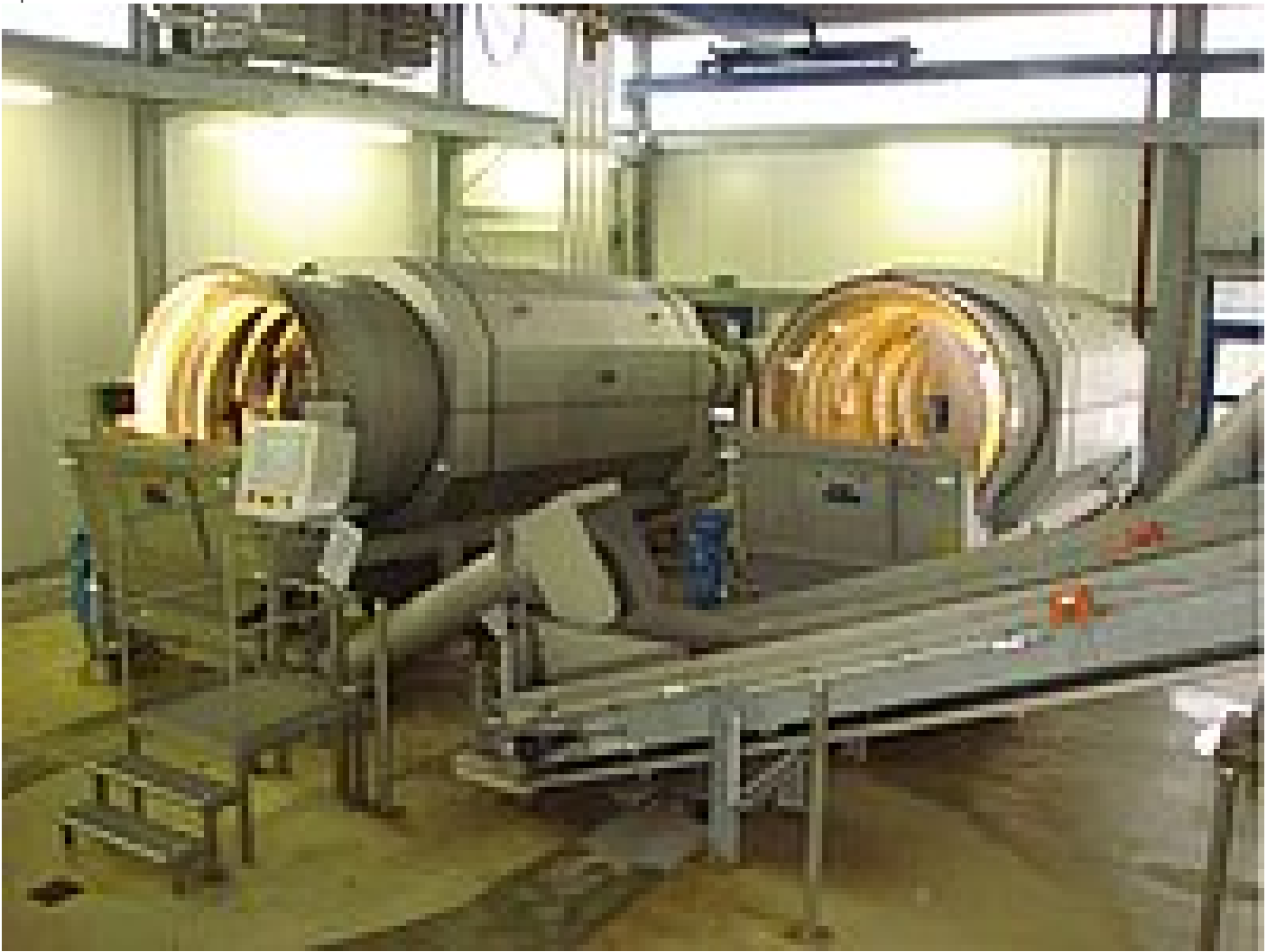
Two ROSF 9 wash drums with WAP screenings presses for the removed and washed coarse solids
