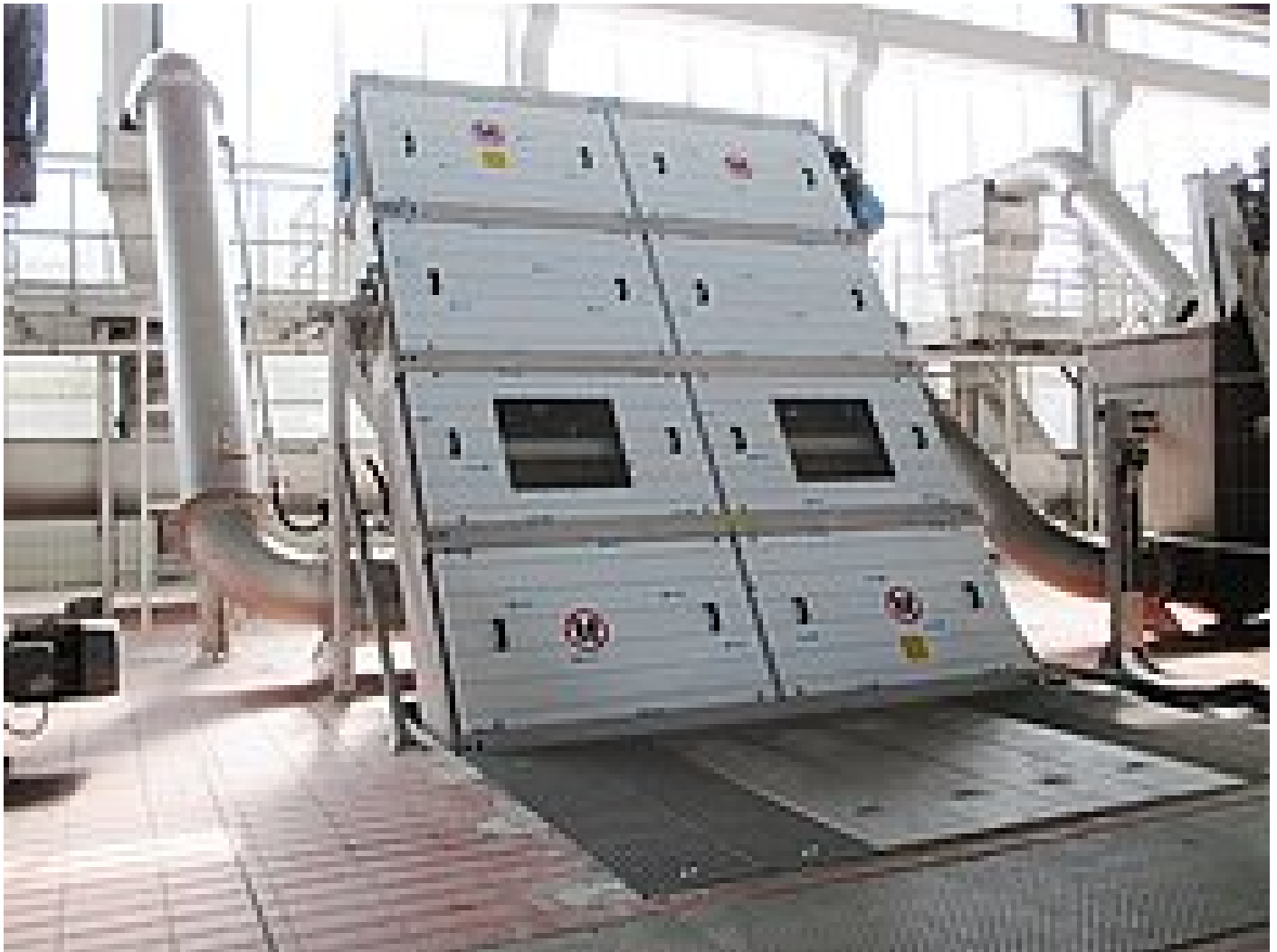
One of the broad HUBER Multi-Rake Bar Screen RakeMax® units with 8 mm bar spacing used as coarse screens
