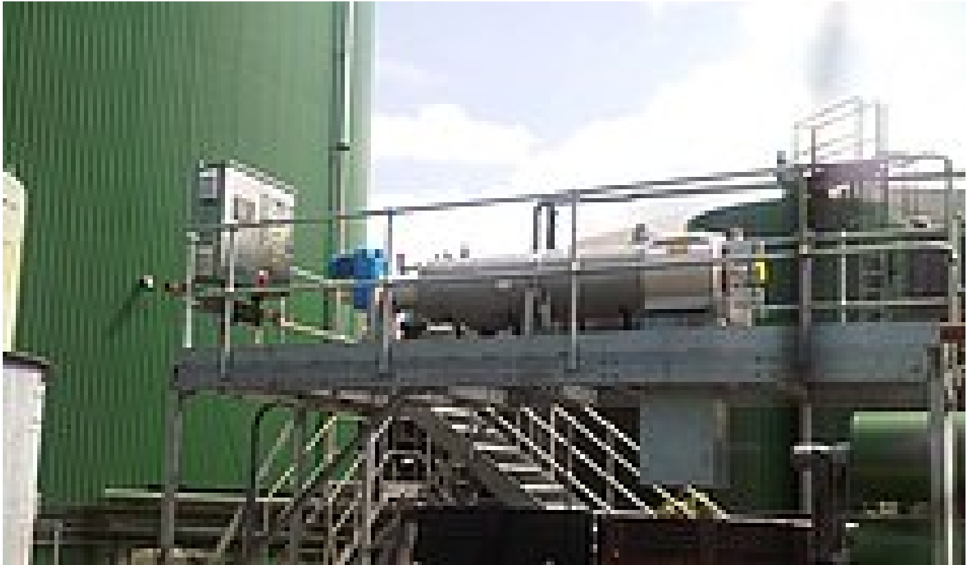
Figure 1: STRAINPRESS® Sludgcleaner on Gantry between digester and first digestate storage tank
